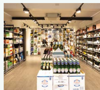
Nolan's supermarket in Ireland installs the first Panasonic CO 2 Condensing Units for showcases. Ireland. Refrigeration
